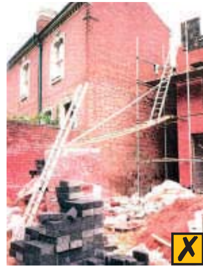
2.0 Highly dangerous practices involving the use of ladders.
