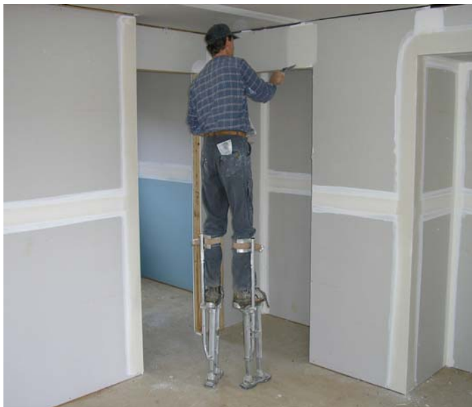
Correct use of stilts: A light duty task being conducted on a clean floor.
